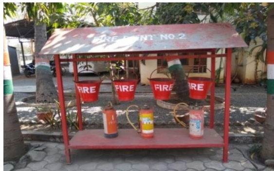
Fire extinguishers with sand buckets
