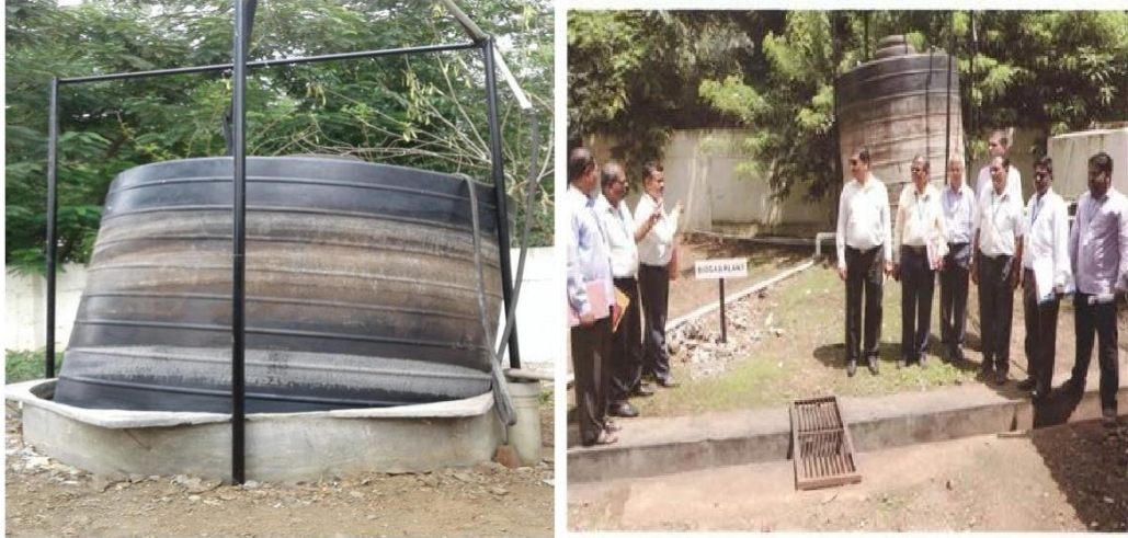
Biogas digester near boy's hostel
