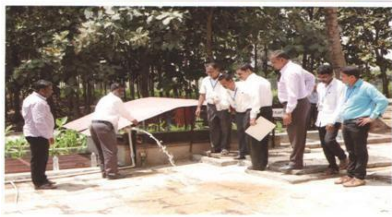
Gray water treatment plant of 40 thousand liters per day capacity
