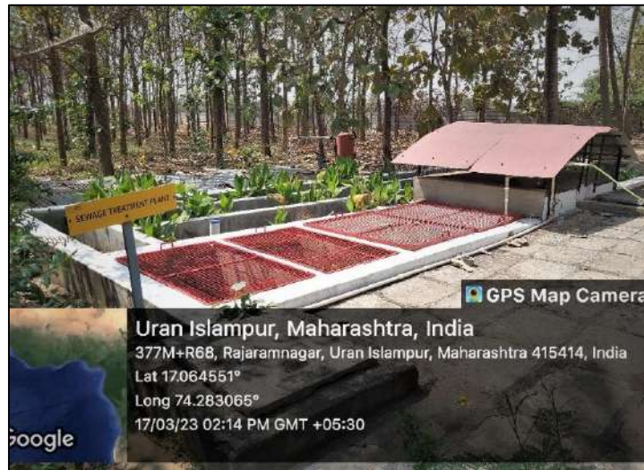
Fig 1: Grey Water Treatment Plant at Boys Hostel
