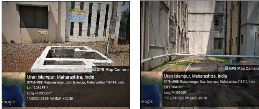
Fig 5: Rainwater harvesting units at Boys Hostel
